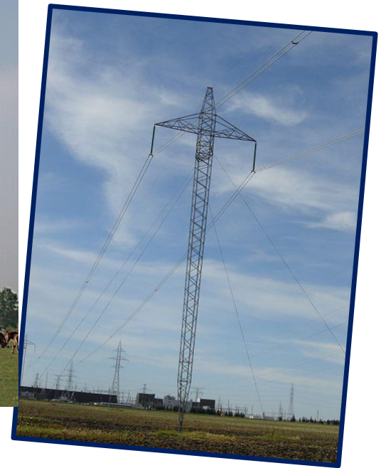
Upgraded electricity grid
